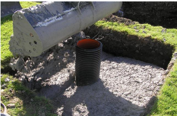
Installation with sockets
